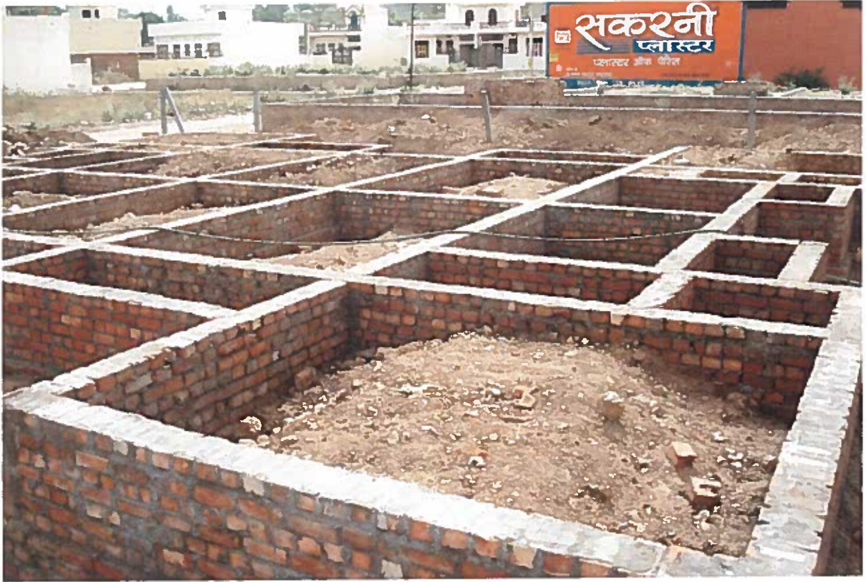
Demonstration Housing Project being constructed by BMTPC at Pinjore, Distt. Panchkula, Haryana
